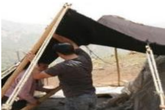
Fig 43. Pulling up the end and the middle column which carries a ridge beam (Source: Author)
