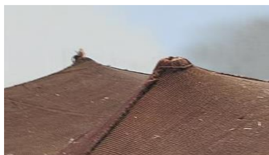
Fig 27. Kormanj Tribe. The outside of the roof holes, where the tips of columns stick out (Source: Author)
