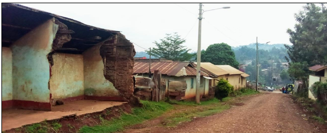
Fig 6. A residential building demolished in Daraja Mbili for illegally being on a road reserve
