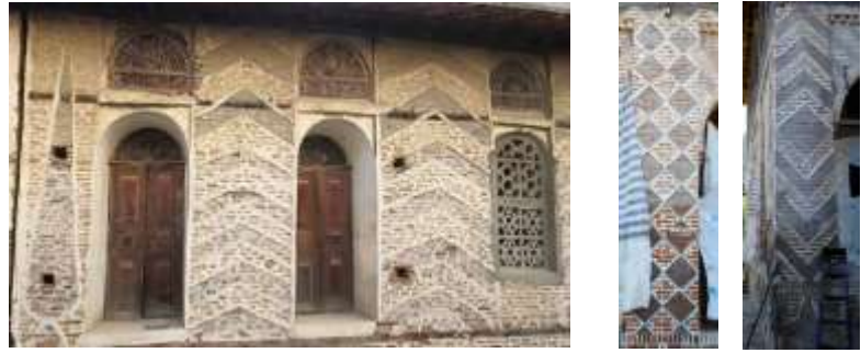
Fig 8. Plasterworks. Left: triangular arches and a cypress motif (Ghoreishi house), center: rhombus pattern (Siami house), right: triangular arches and rhombus (Siami house)
