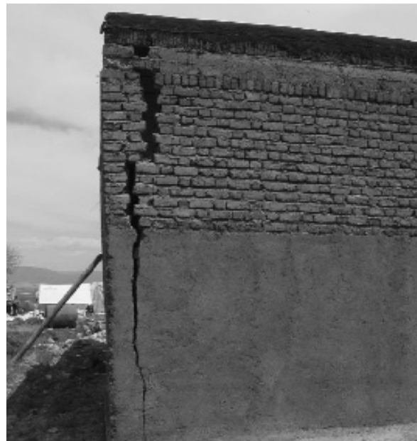
Fig. 1 Vertical crack in confined masonry wall due to out-of-plane action of other wall during Silakhor earthquake
