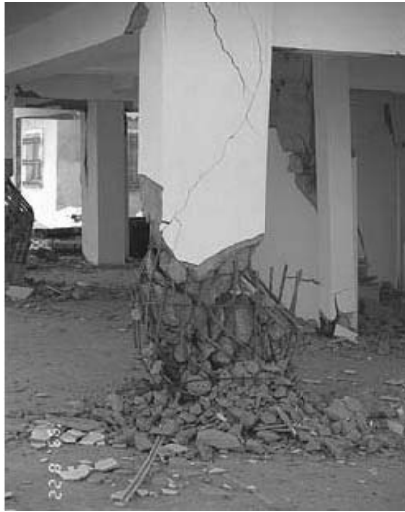
Fig.1 Failure of lap splice due to widely spaced ties with 90° hooks (Izmit-1999)
