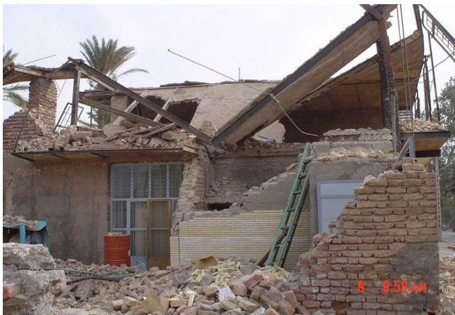
Fig. 4 Damaged buildings, combination of steel internal columns and load-bearing external brick-walls
