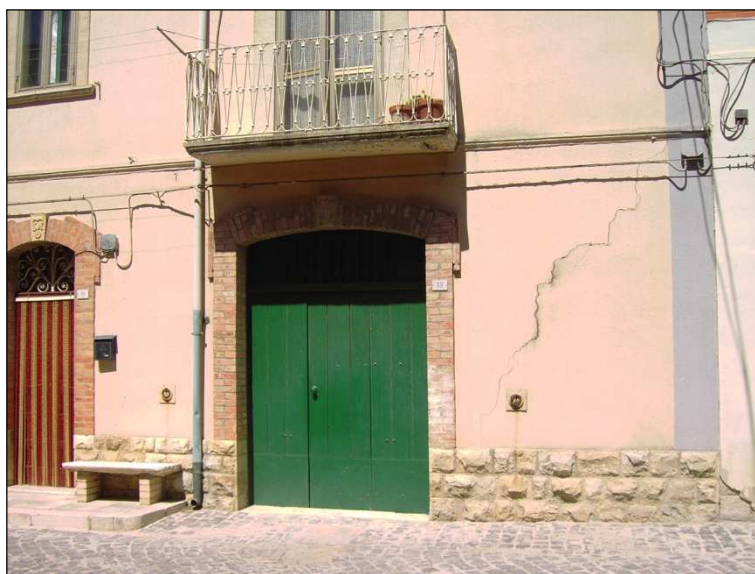
Fig. 36. Half arch-shaped crack on a building in Pietramontecorvino (Puglia, Italy)
