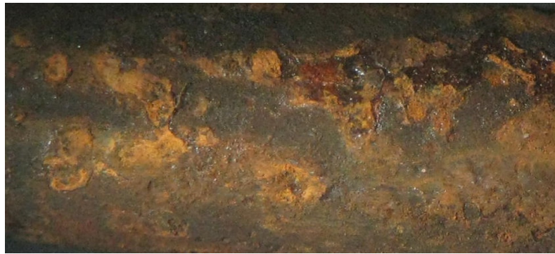
Fig. 5. A view of eroded contact
