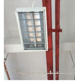
Fig 1. Actual figure of lighting fixtures
