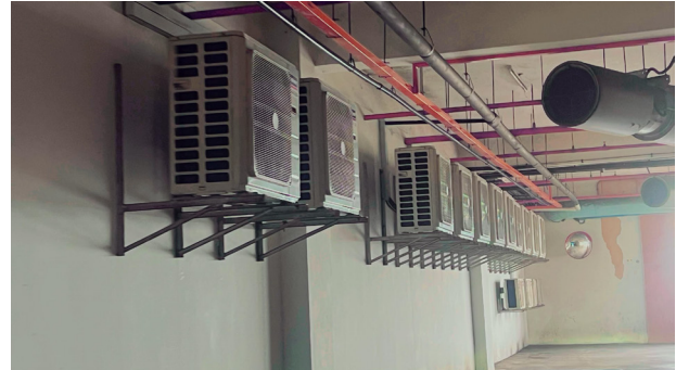
Fig. 1 A group of condenser units installed outside a management building in Kuala Terengganu, Malaysia.
